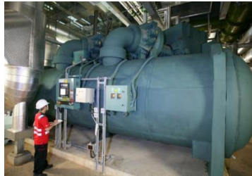
Photo: Kai Tak's district cooling system using seawater from the Kowloon Bay.
